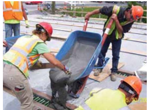
Fig. 7: Longitudinal connections cast between deck-bulb-tee girders. Field cast UHPC can simplify connection details and construction (NY DOT), Source: [1]
